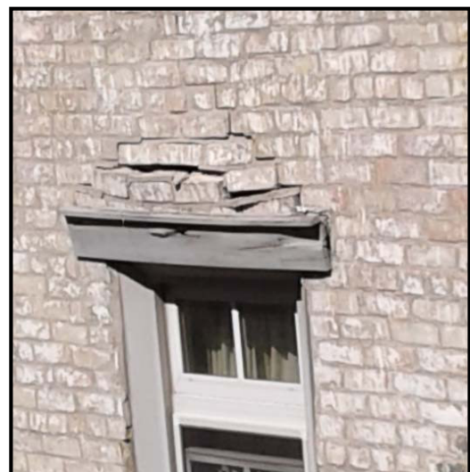
Window needing repair at 411 N Center
