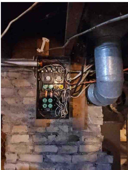
Basement - Older Turn Fuse
