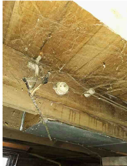
Basement - Some Knob & Tube Wiring
