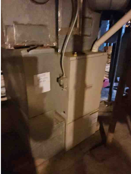
Basement - Older HVAC
