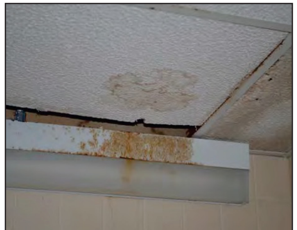
Right: Water damaged ceiling tiles inside of the Creativity Center.
