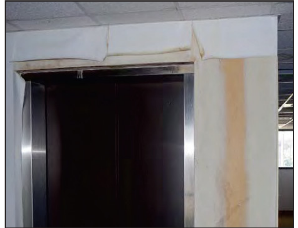
Right: Water damage around the elevator in the Creativity Center.
