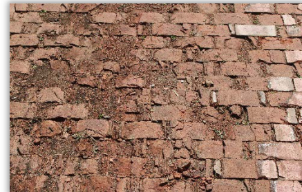
Figure 15: Patio paver bricks after years of use
