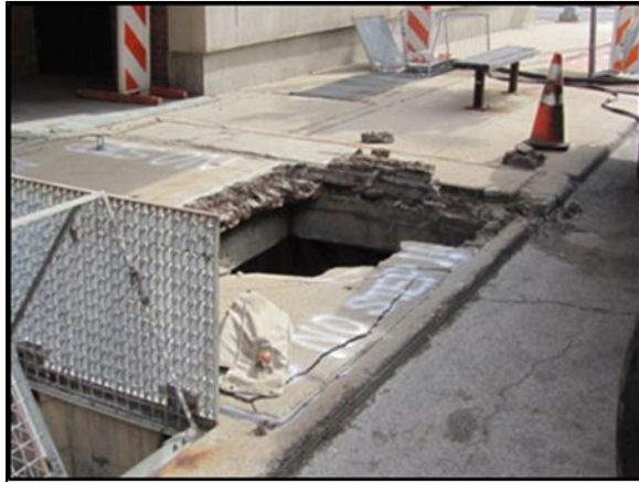
Figure 10: A Collapse Sidewalk Above a Vault
