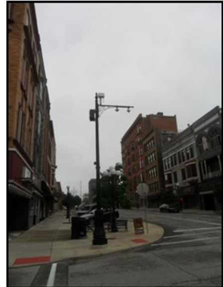
Figure 7: Camera & Wireless Access Point Pole Example
