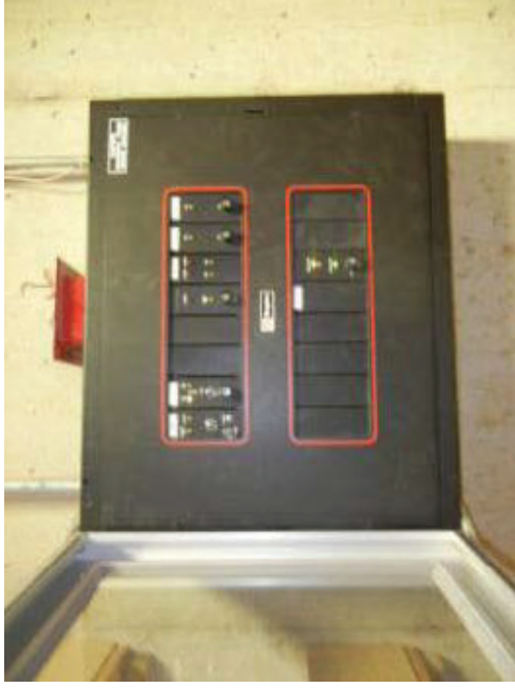
Old / Obsolete Fire Alarm Systems – Various Facilities
