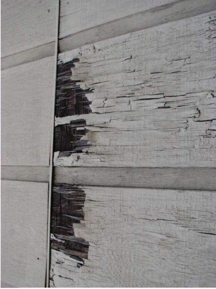
Severely Deteriorated Siding at Public Works Garage
