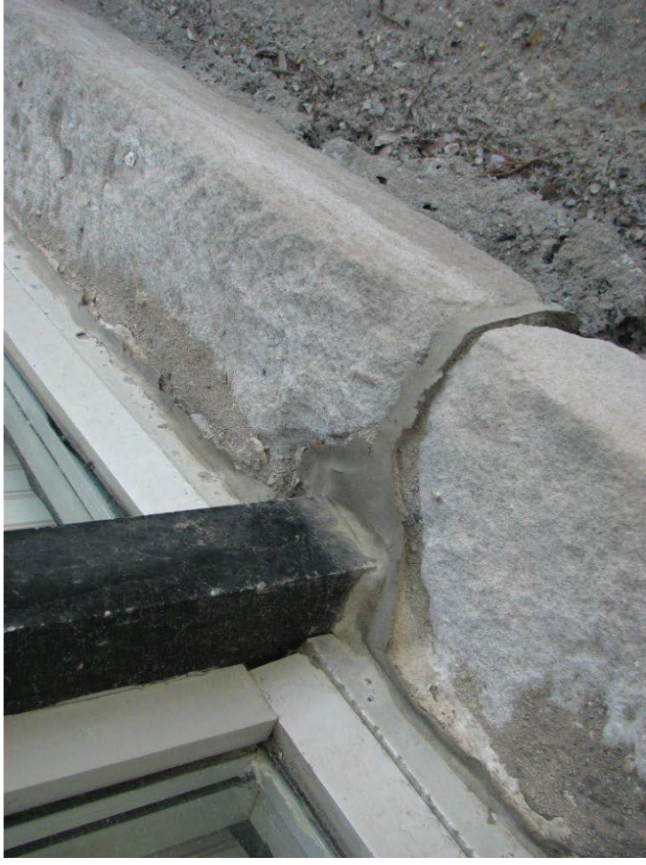
Window Sill Deterioration at City Hall
