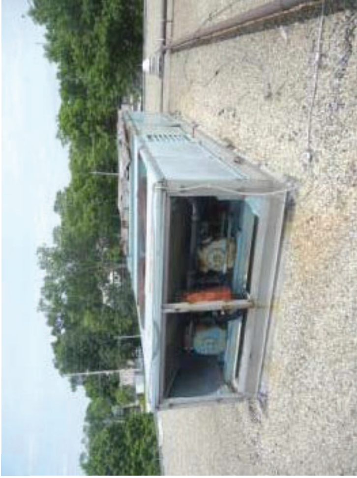
Old / Obsolete HVAC Systems – Various Facilities
