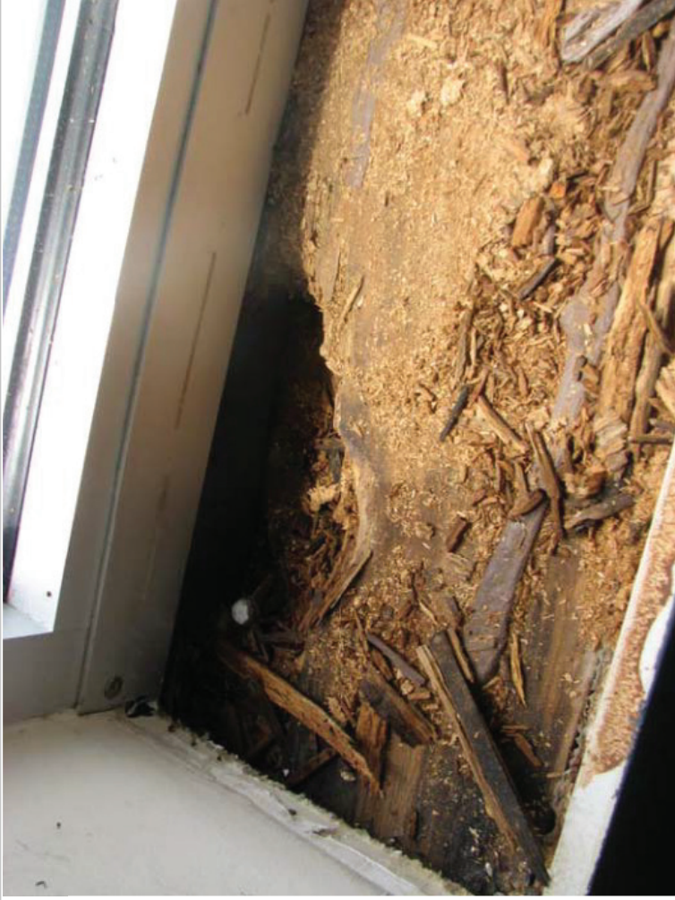
Water Damage at Police Department Administration Office
