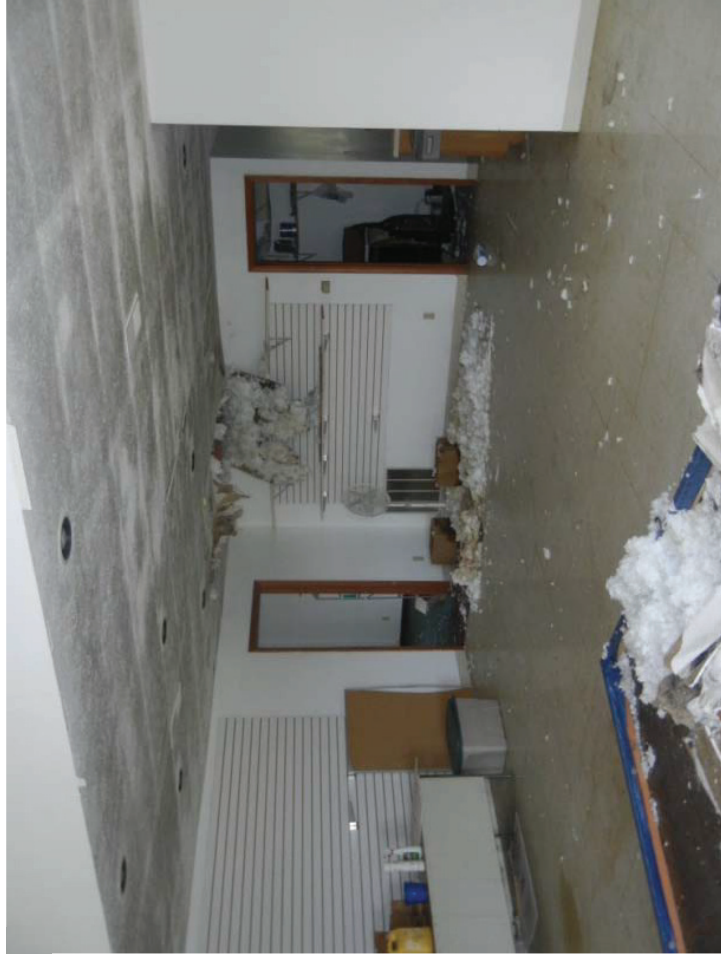
Water Damage in Police Training Facility Lodge
