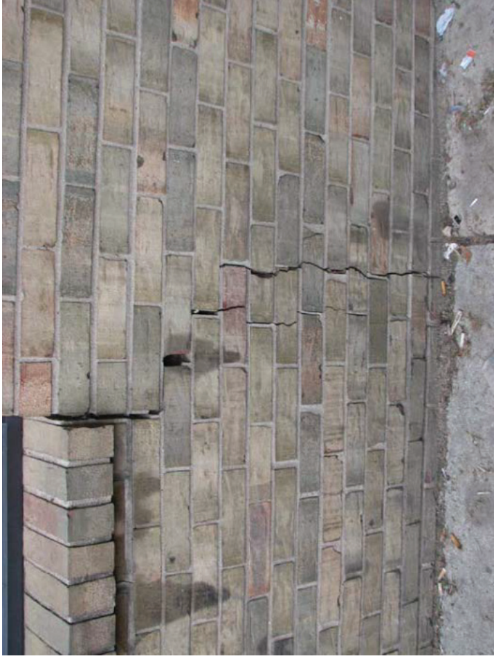
Deteriorated Wall at Public Works Garage
