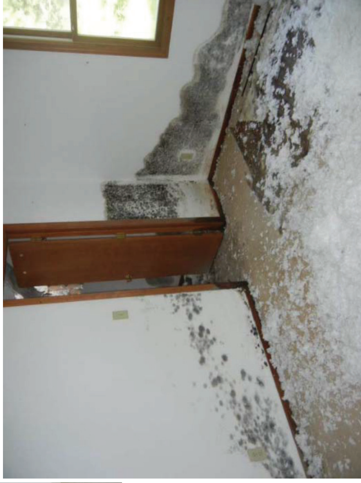
Mold Damage in Police Training Facility Lodge
