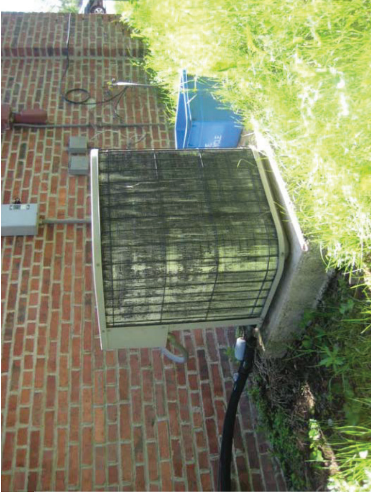
Old / Obsolete HVAC Systems – Various Facilities
