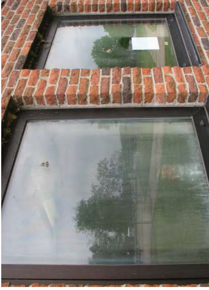
Failed Windows at Water Treatment Plant
