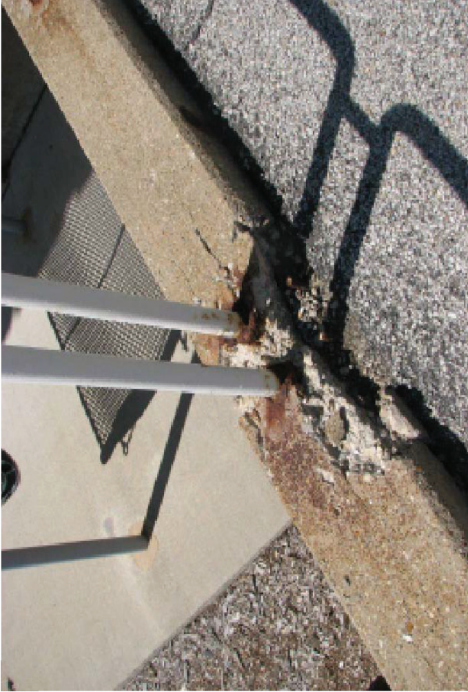
Ramp and Wall Deterioration at City Hall
