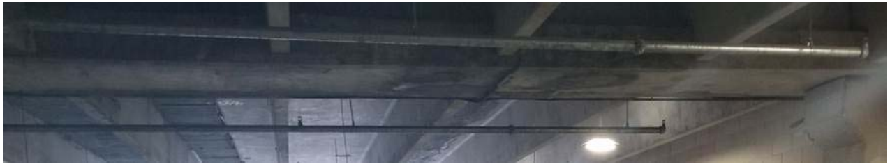
BEAM PRIOR TO LOOSE CONCRETE REMOVAL
