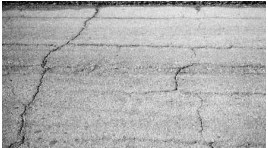
▼ Block cracking with open cracks.
