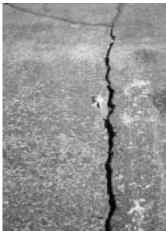
▲ Open crack – 1/2" or more in width.
