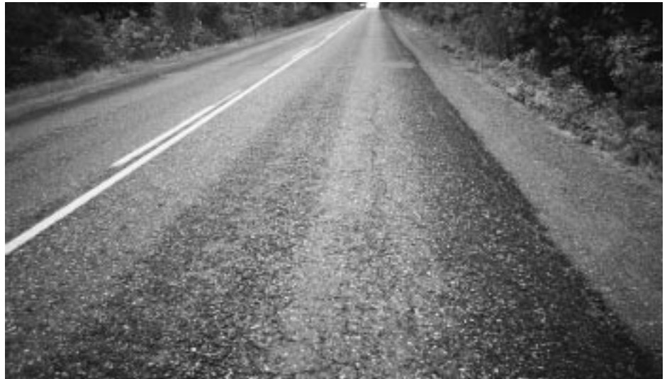
► Moderate to severe raveling in wheel paths.
