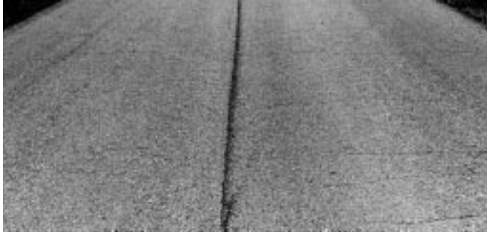
Centerline crack (still tight). ▶
