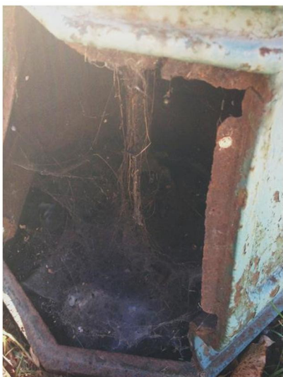
Figure 4 – Interior deterioration shown in one of the 12 decorative pole bases.
