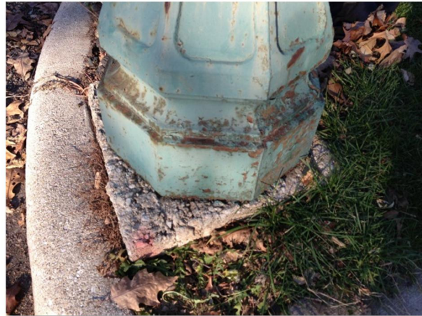
Figure 3 - An existing concrete foundation deteriorating beneath a pole base.
