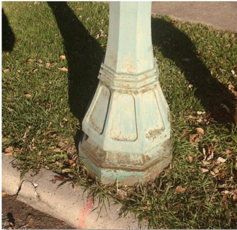
Figure 2 - An existing pole base foundation shown sunk into the soil allowing increased weathering around the base.
