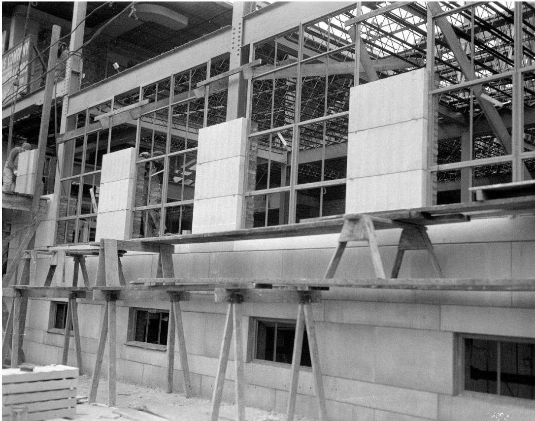
Photo Credit: Bill, Frank; Pantagraph Building construction, Bloomington, IL, 1935, Pantagraph Negatives Collection (Illinois Digital Archives), 2025-06-21, http://www.idaillinois.org/digital/collection/p16614coll35/id/4616 .
