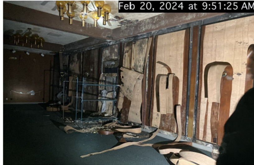
Water damage (including at least some identified structural damage)
