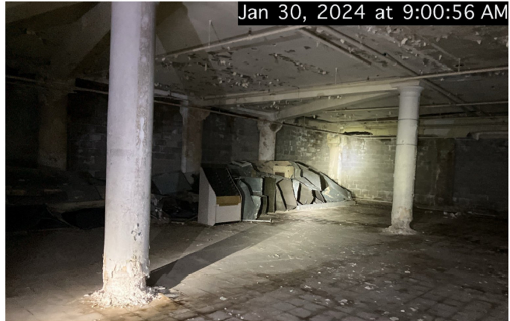
Damage to structural support system; throughout
