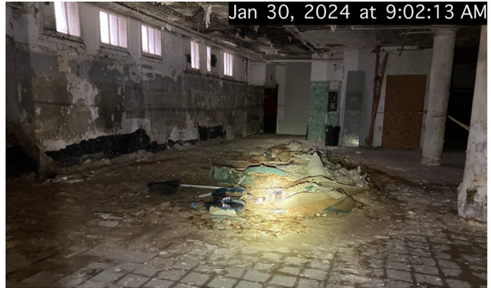
Generalized deterioration and evidence of water infiltration issues
