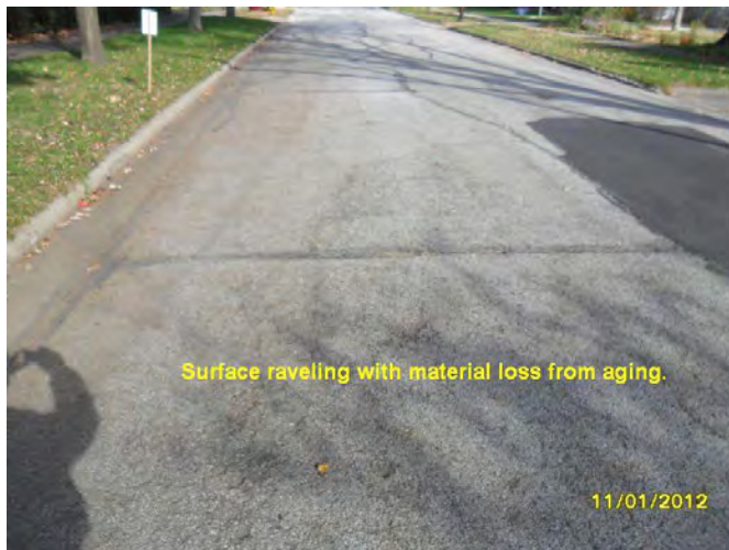
Figure 6 - Moore Street prior to 70/30 CRF treatment
