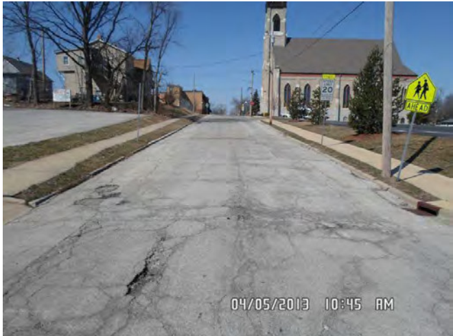
Figure 8 - Jackson Street prior to CRF treatment
