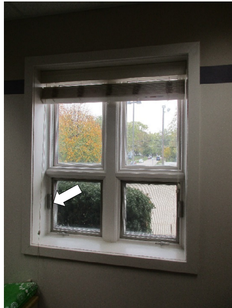
Figure 4: Operable window controls
