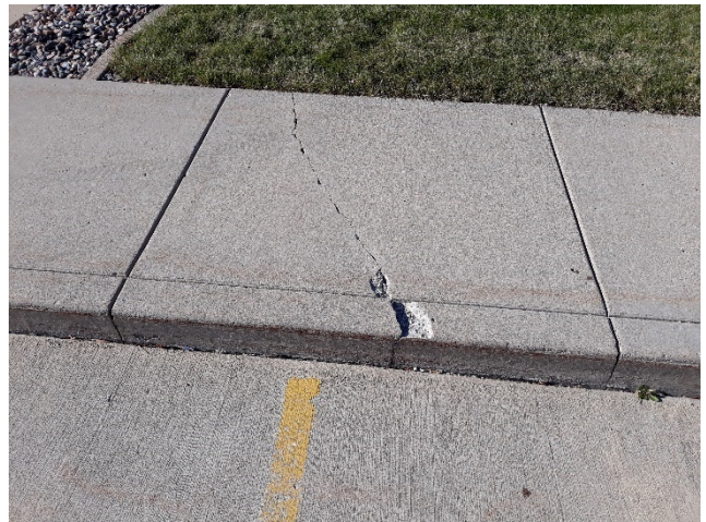
Figure 26: Crack in concrete walk
