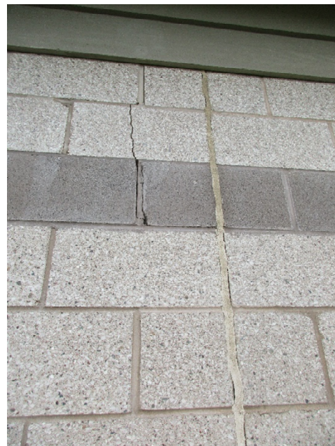
Figure 10: Cracked mortar and block near control joint
