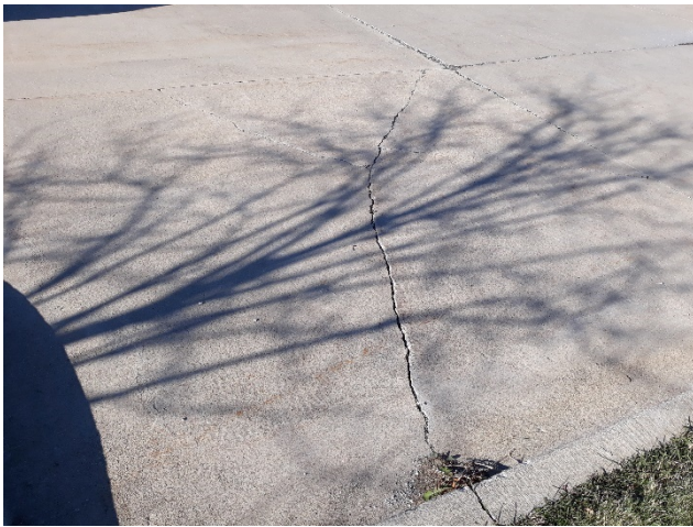
Figure 25: Cracks in concrete drive
