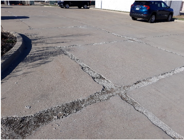
Figure 29: Spalling at concrete drive joints
