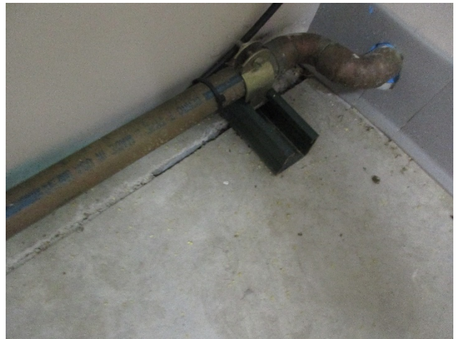
Figure 22: Floor gap Mech 126
