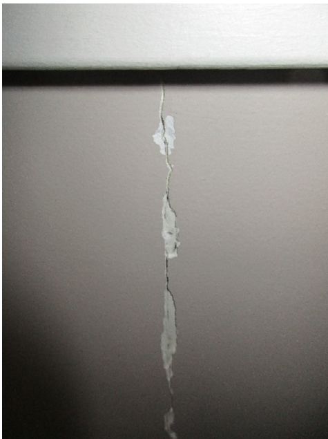
Figure 19: Below window at Break 121
