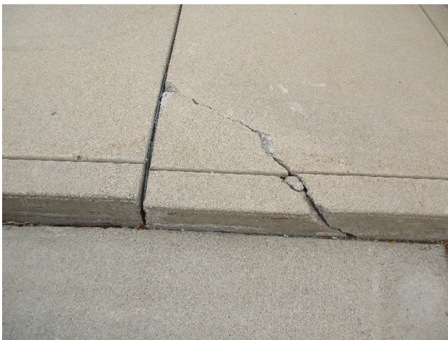
Figure 27: Crack in concrete walk
