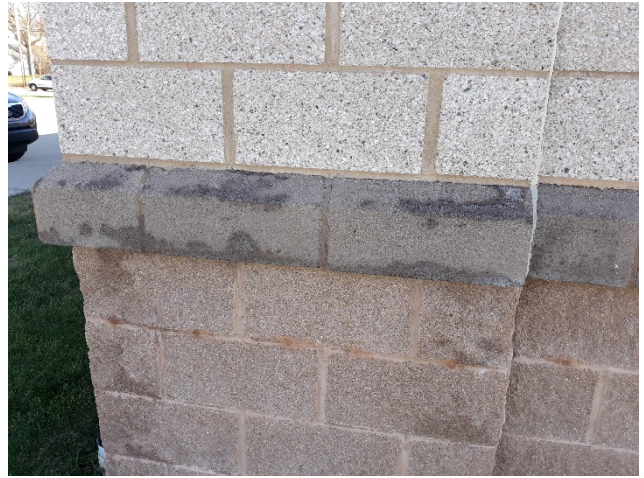
Figure 12: Discoloration of precast band and masonry
