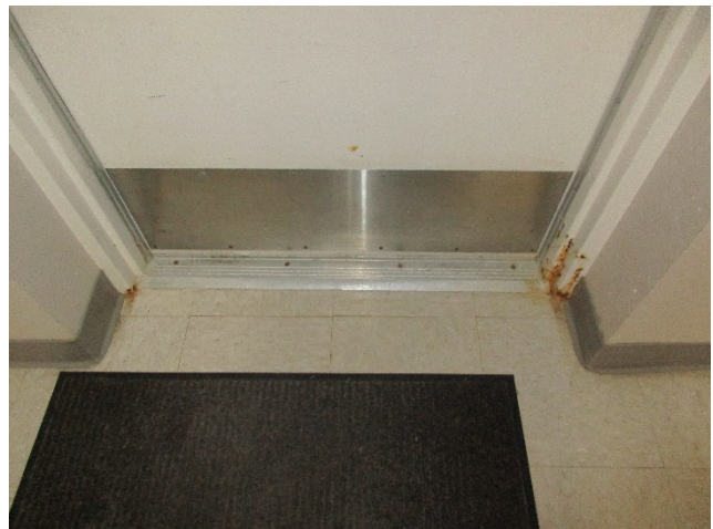
Figure 14: Rust at bottom interior of HM door
