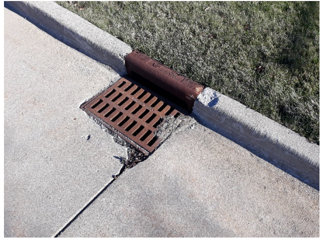
Figure 30: Spalling of concrete joint at inlet
