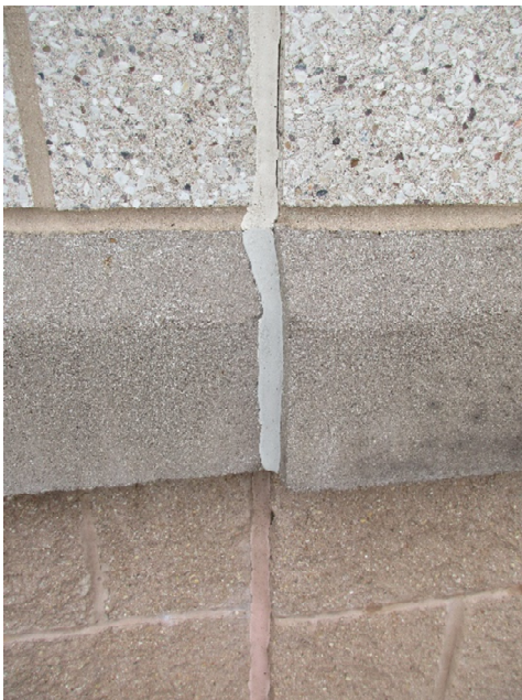
Figure 9: Sealant at control joint
