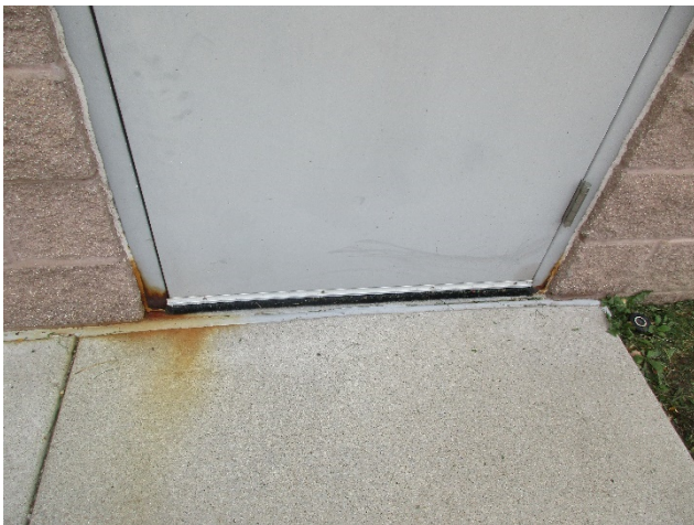
Figure 15: Rust at bottom exterior of HM door
