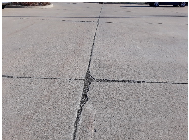
Figure 28: Spalling at concrete drive joints
