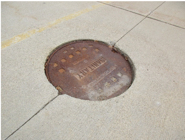
Figure 31: Depressed manhole cover
