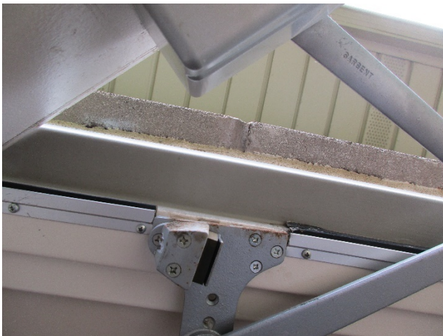
Figure 13: Discontinuous weatherstripping at door closer
