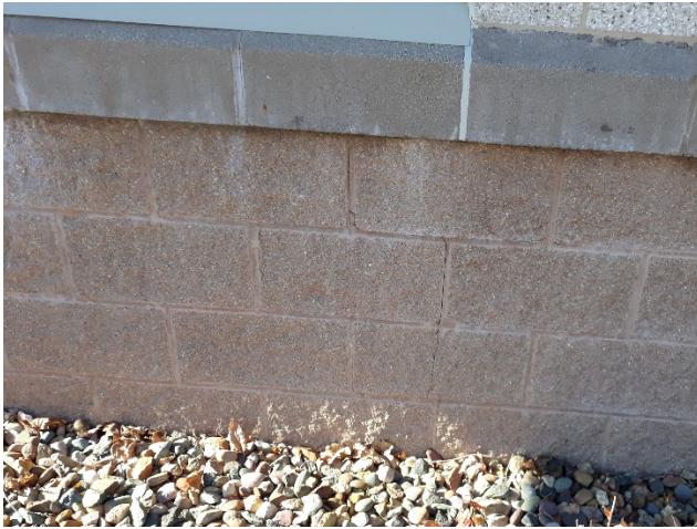
Figure 11: Cracked mortar joints and block
