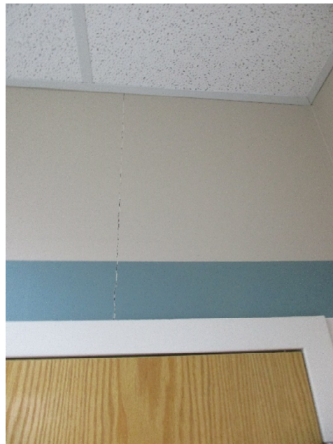
Figure 20: Above door at Office 133
