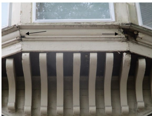
Both of the outer corners on the lower crown trim below the rest bump out showed wear/rot that will need repair to ensure no further water leakage into the woodwork
