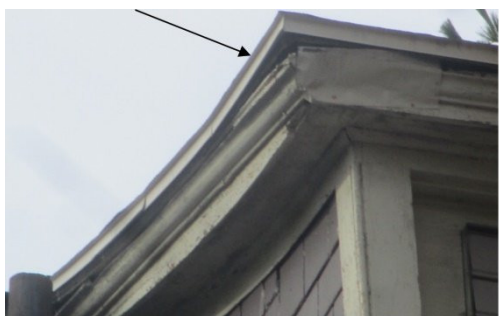
Corner areas on the back dormer on the roof are showing small pen area that should be properly sealed to prevent pests access to the inner attic space area
