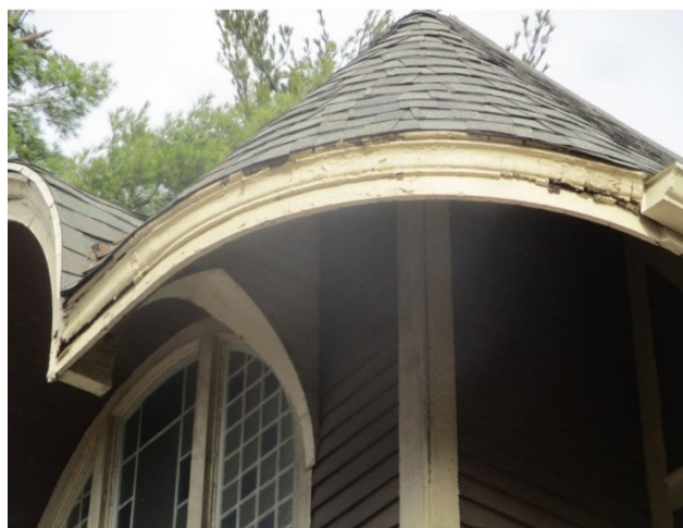
Wear areas on the front upper fascia band on the front SE corner of the home that is in need of future repair
