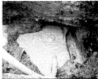
Hidden leak running into drain tile
