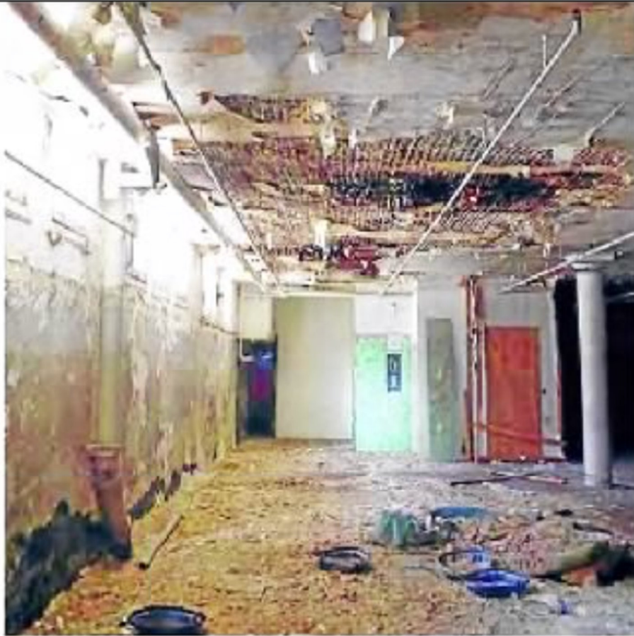
PGAV PLANNERS, FOR THE PANTAGRAPH Water damage can be seen inside the Front 'N' Center building in Bloomington.
