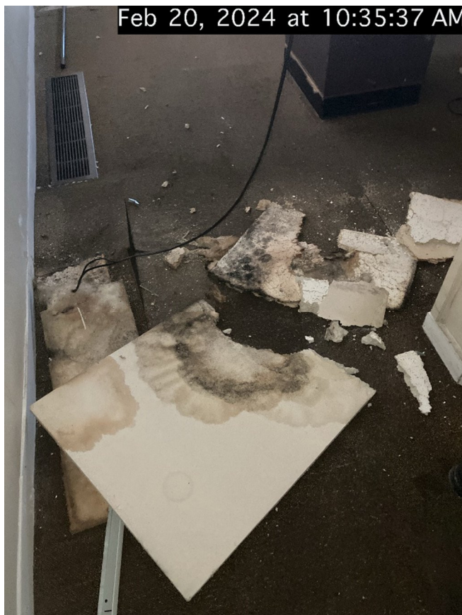
Generalized mold/mildew contamination throughout the building.
