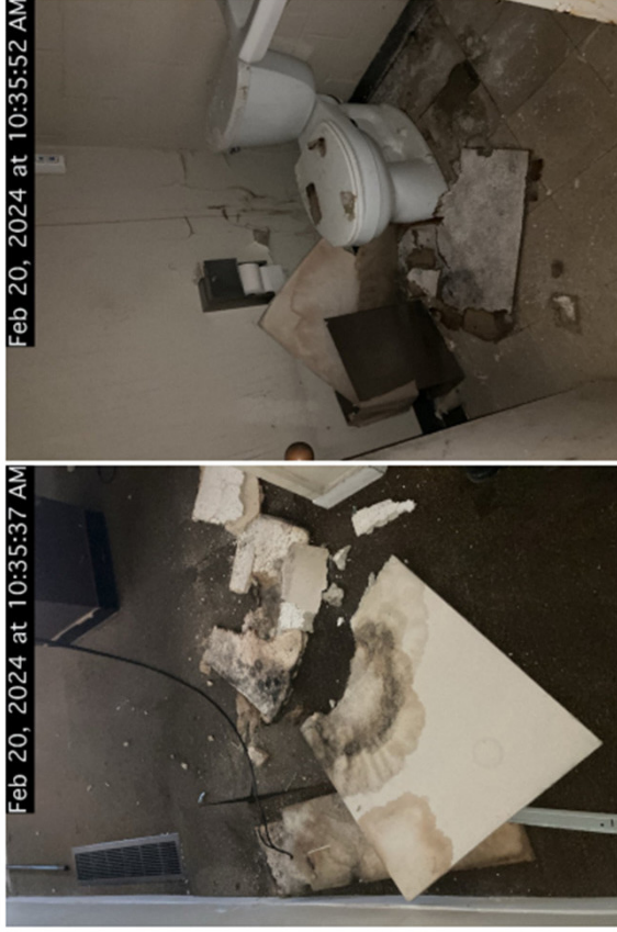
Generalized mold/mildew contamination throughout the building.
