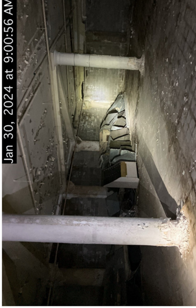
Damage to structural support system; throughout
