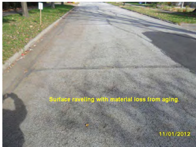
Figure 6 - Moore Street prior to 70/30 CRF treatment
