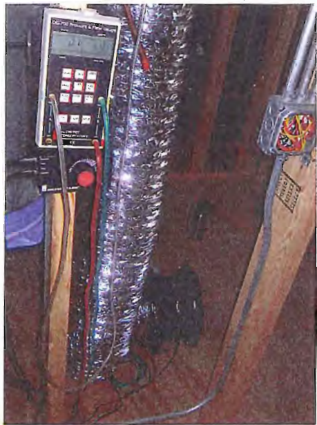
This is a Rough-in Total Leakage test, without the air handler installed. The blower and manometer are the only equipment required
