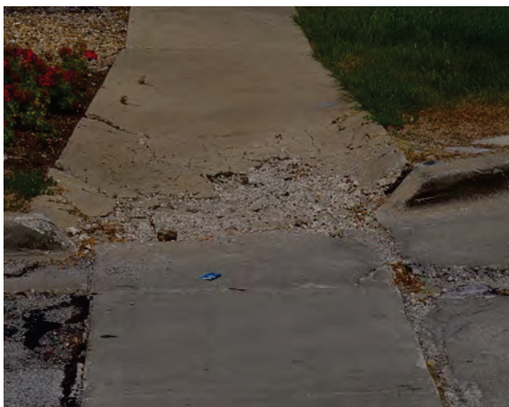
Left: A deteriorated sidewalk along IAA Drive.
