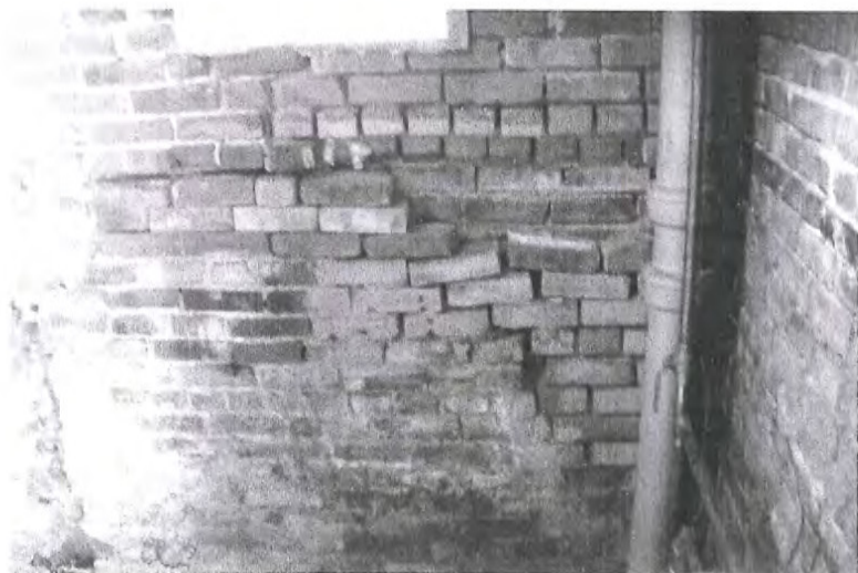
BROKEN & REMOVED BRICK
