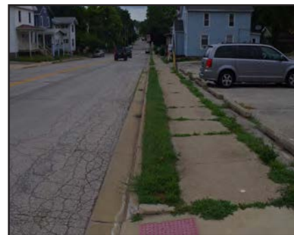
Below: Deteriorated pavement along North McLean Street.
