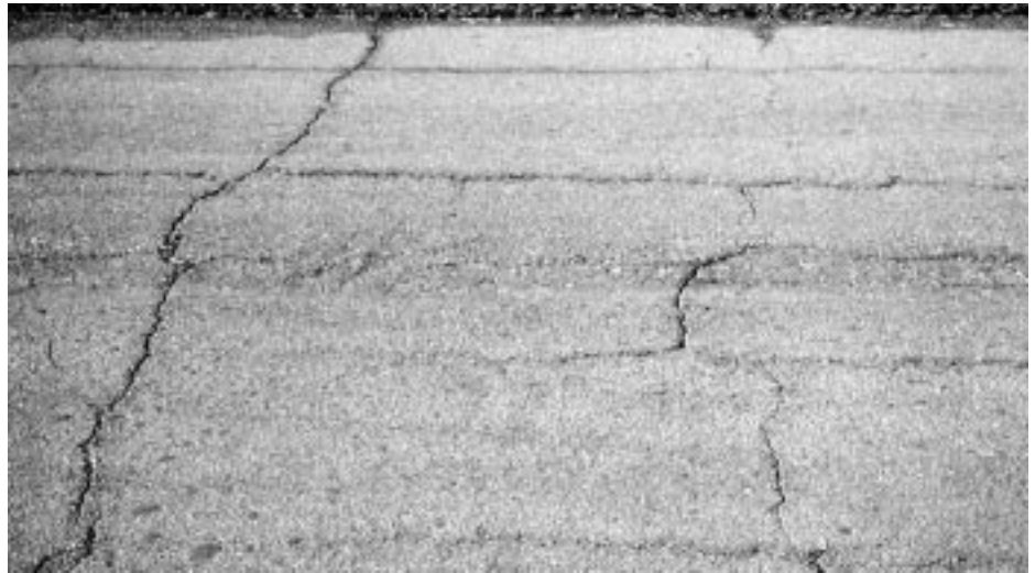
▼ Block cracking with open cracks.
