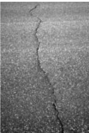
▲ Tight cracks less than 1/4" in width.
