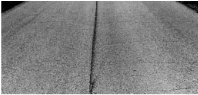
Centerline crack (still tight). ▶
