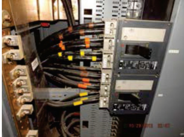
Figure C-2: Ice Plant Breaker
